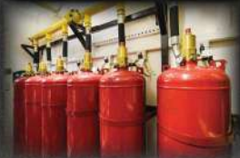
Fire alarm system
